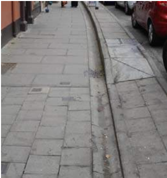
Numerous level changes impede pedestrian flow.
