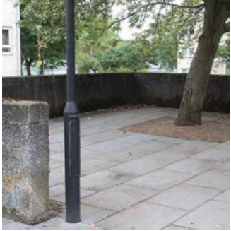
Right: Rendered concrete walls create unused isolated spaces between the Vennel and High Street.
