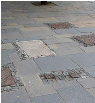
Left: Poor quality implementation and attention to detail detracts from quality of materials and leads to potential trip hazards
