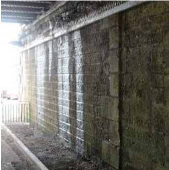
Poorly lit, unsightly and uninspiring underpass leading to Station Road immediately adjacent to train station exit.
