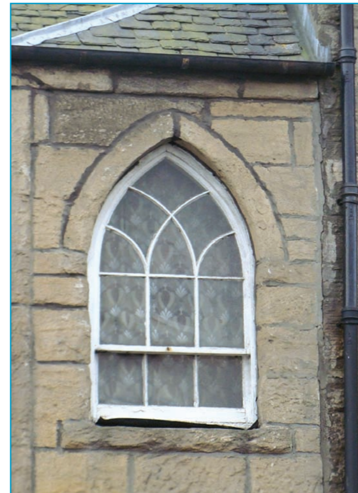
This sash window required skilful workmanship, and was probably constructed by a freeman of the Linlithgow Incorporation of Wrights.
